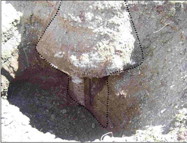
In this excavated foundation, note the overbreak approximately 1 m below the ground line.
