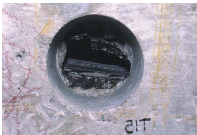
Figure 1. Tendons exposed by Diamond Overcoring
