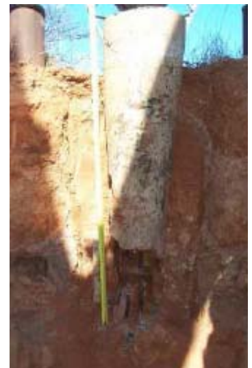
Voiding in tower foundation detected by NDT methods
